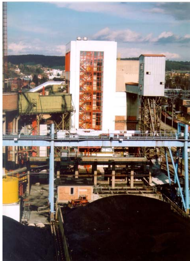
A look at the boiler room of the boiler with CFV 125 t/h Moravské teplárny Zlín
