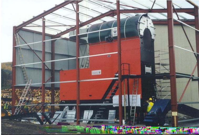
Figure 2 3 MW th wood-fired boiler, located in Scotland, used for heating of drying kilns
